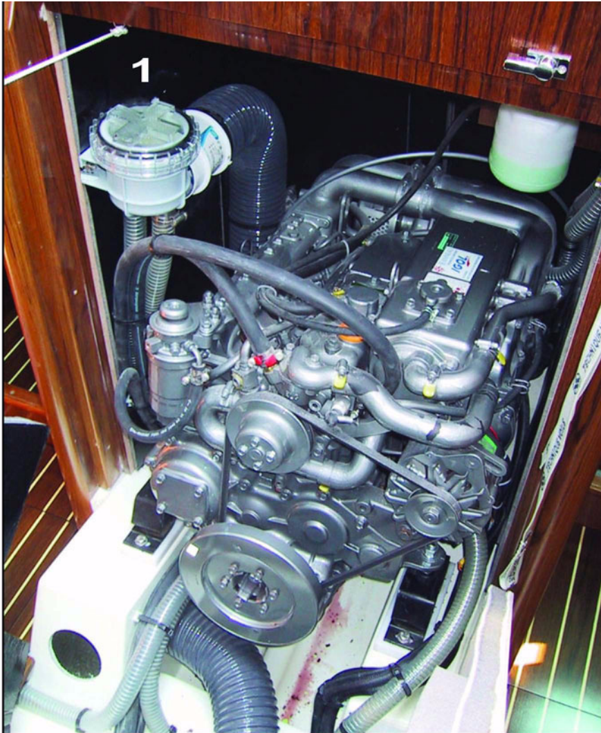
1. Filter for engine cooling water
